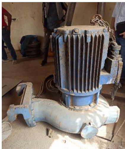
Figure 10 | Low Efficient and Nonoperating Pump, (© IfaS)
