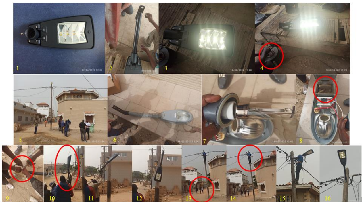
Figure 26 | Images of the Installation Steps of a Prototype of the Lanz Luminaire in February 2022 in the Diamaguène District of Saint-Louis, (© IfaS)
