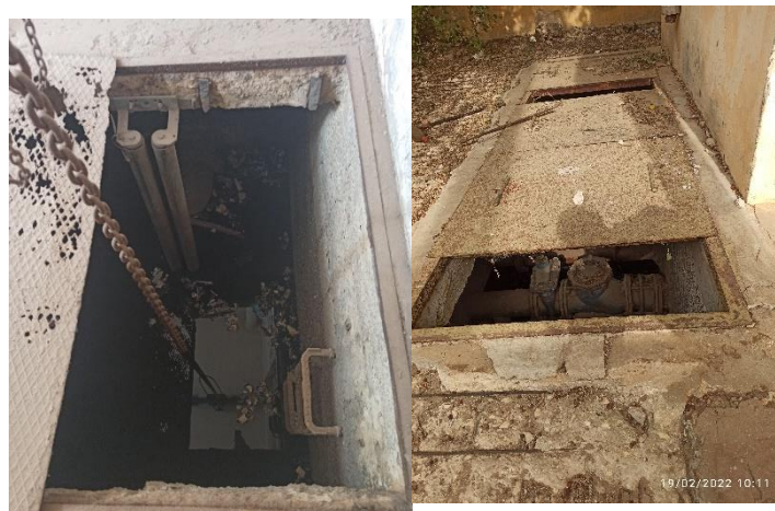
Figure 8 | Pumping Station SP14, (© IfaS)
