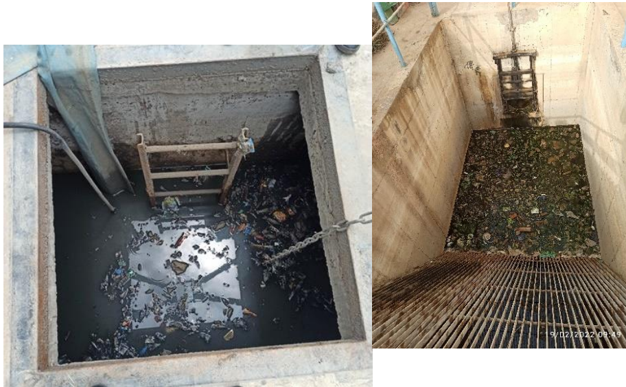
Figure 9 | Discharge chamber of Leona (Right) and Goxu Mbacc (Left) Pumping Stations station Full of Waste, (© IfaS)
