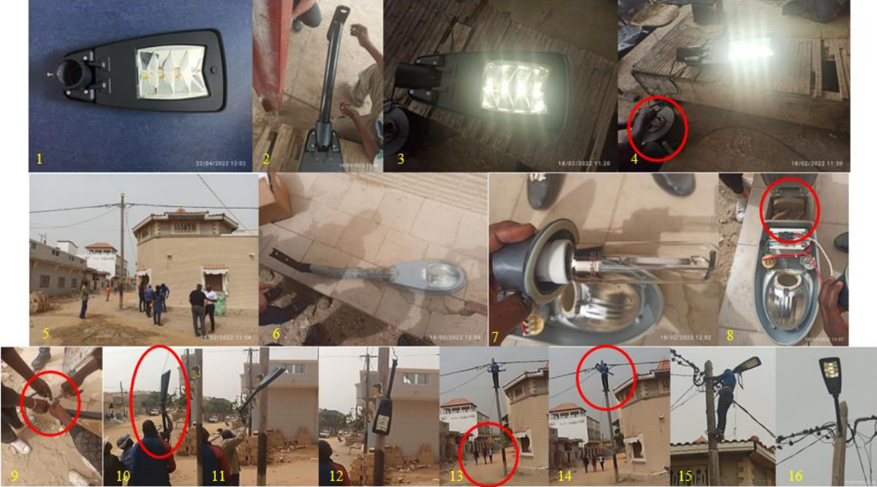
Figure 48 | Images of the Installation Steps of a Prototype of the Lantz Luminaire in February 2022 in the Diamaguène District of Saint-Louis, (© IfaS)
