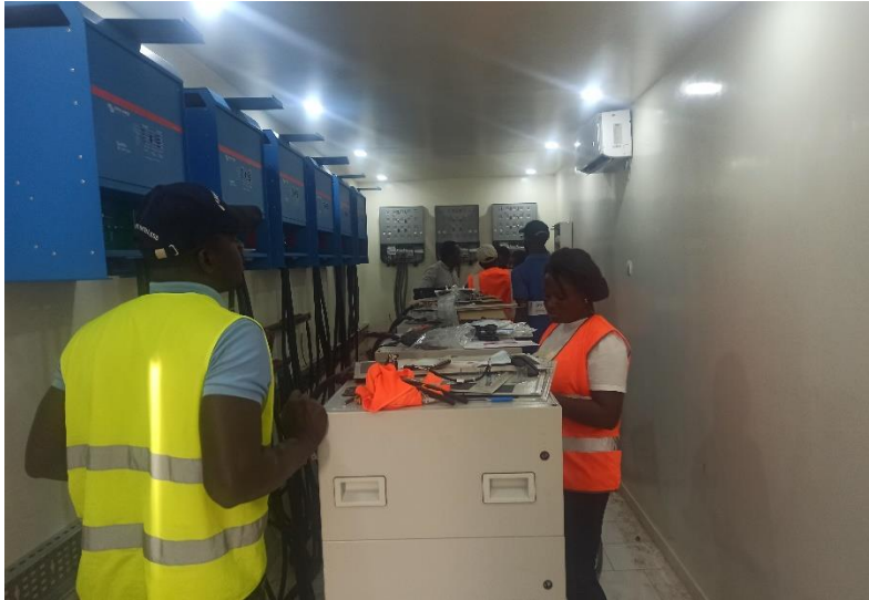
Figure 9 | Technical Chamber of PV Plant at UGB with the Participation of Students and Technicians, (© IfaS)
