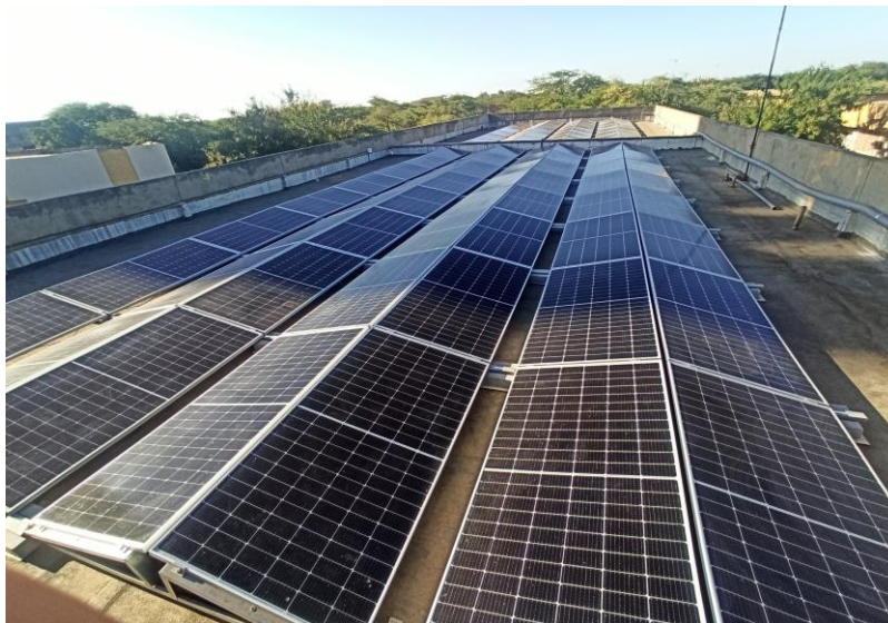
Figure 8 | PV Plant Installed in Building A at UGB, (© IfaS)
