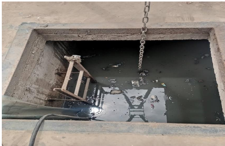
Figure 7 | Leona Pump Station Full of Wastewater, (© IfaS)
