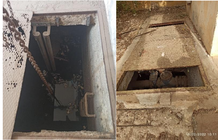
Figure 1 | Pumping Station SP14, (© IfaS)
