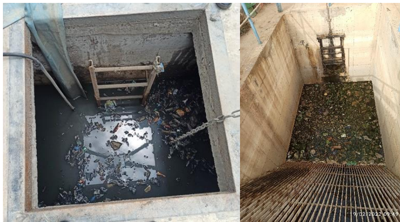
Figure 2 | Discharge chamber of Leona (Right) and Goxu Mbacc (Left) Pumping Stations Station Full of Waste, (© IfaS)
