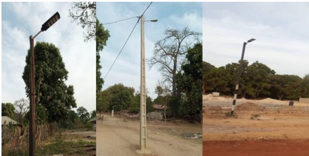
Figure 5 | Presently available Streetlight Systems, (© IfaS)
